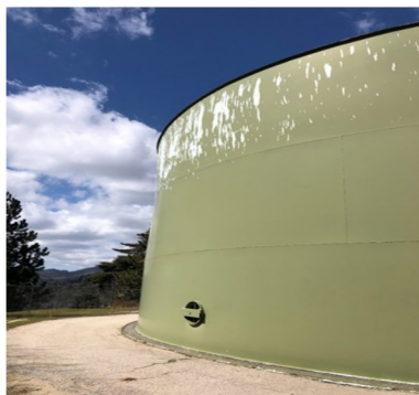
Brookside Wells Figure 3 SCADA & Data Collection, outside coating should be evaluated
