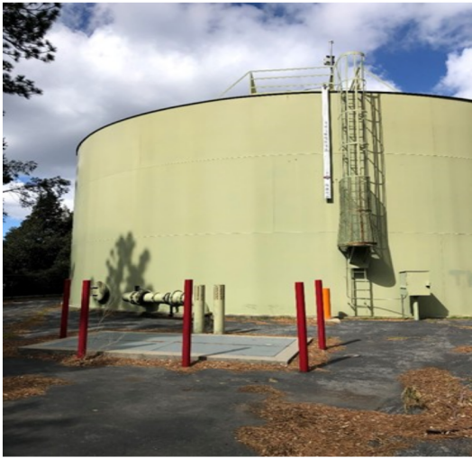
Figure 1 - Old Mill Tank - Just SCADA - some outside coating failures
