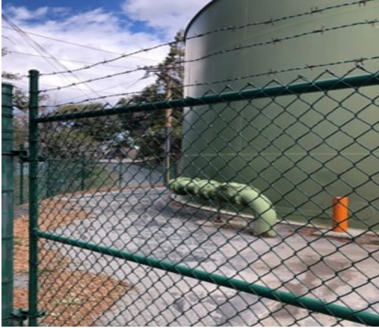
Figure 1 - CLAVAL PRV station (Hydraulically controlled), SCADA and data collection
