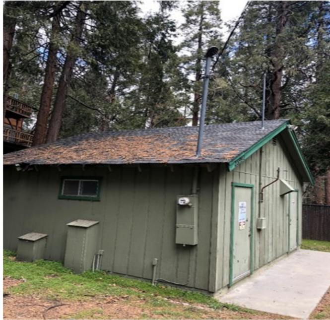
Pioneer Well - 4 horizontal wells, chlorine phosphate and SCADA
