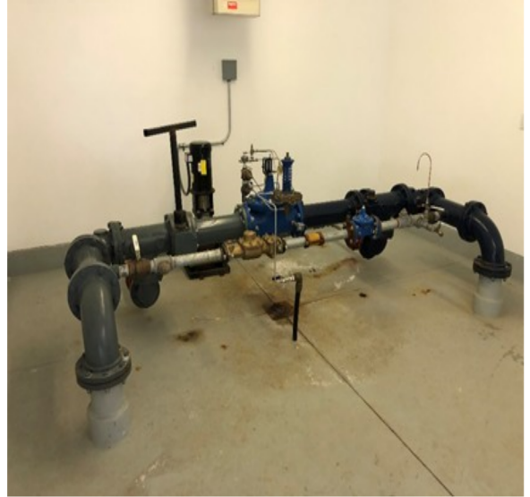
Figure 2 - CLAVAL PRV station (Hydraulically Controlled), SCADA and data collection
