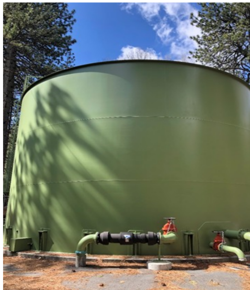
Figure 3 - two tanks SCADA and data collector
