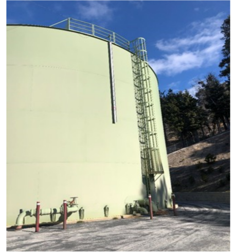
Figure 3 -2 tanks SCADA and Data Collector
