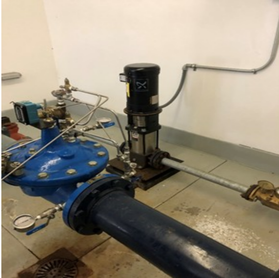
Figure 1 - CLAVAL PRV station (Hydraulically controlled), SCADA and data collection
