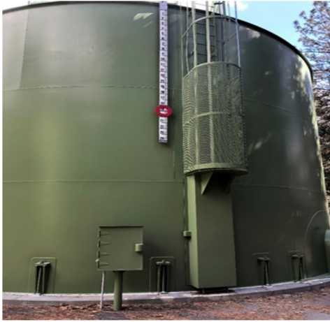
Figure 1 - two tanks, SCADA and data collector
