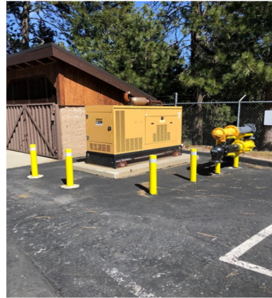
HQ - Emergency Genset Figure 2
