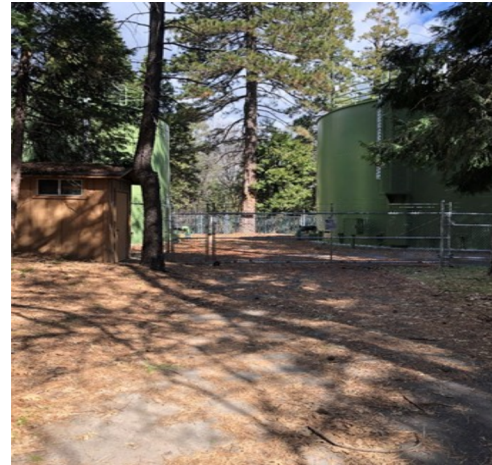
Figure 2 - two tanks, SCADA and data collector
