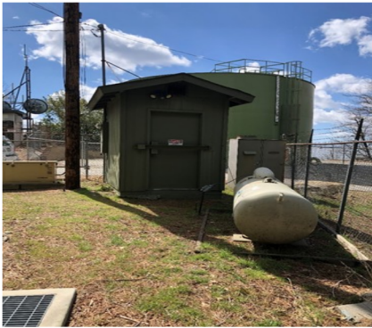
Figure 4 - Beacon I & II, SCADA and Data Collection
