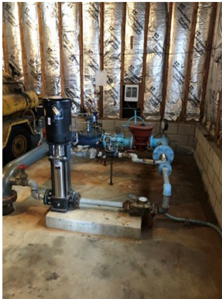
Figure 3 - Barn Tank, SCADA and Data Collection
