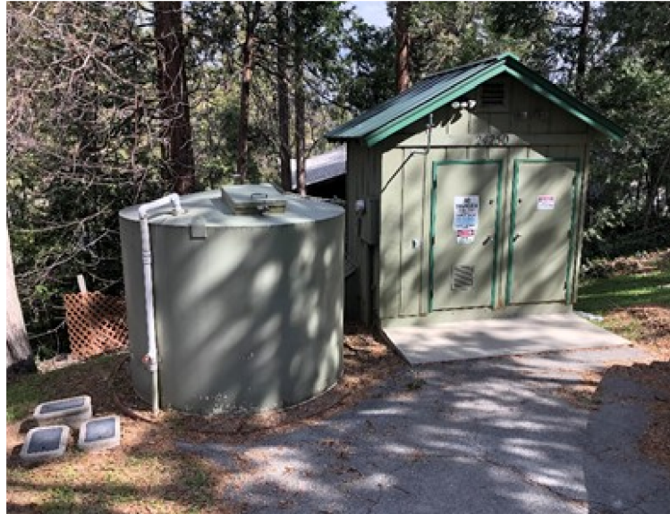
Horst - 3 Horizontal Wells Chlorine and Phosphate and SCADA
