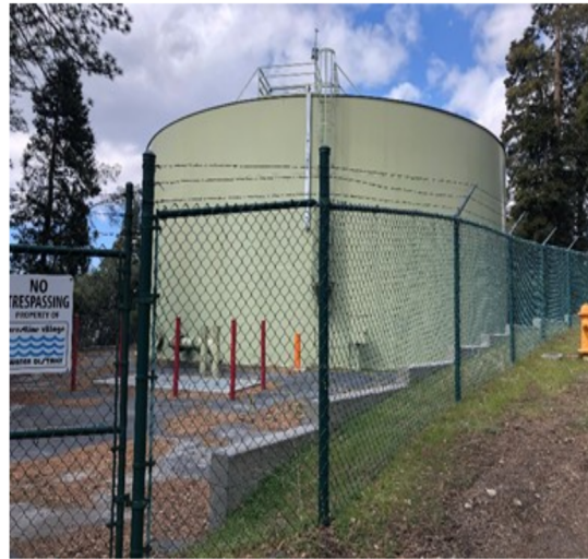
Figure 2 - Old Mill Tank - Just SCADA - some outside coating failures
