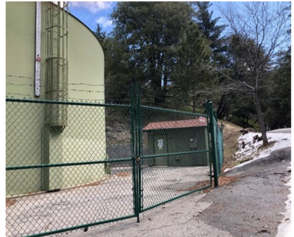
Figure 2 - CLAVAL PRV station (Hydraulically controlled), SCADA and data collection
